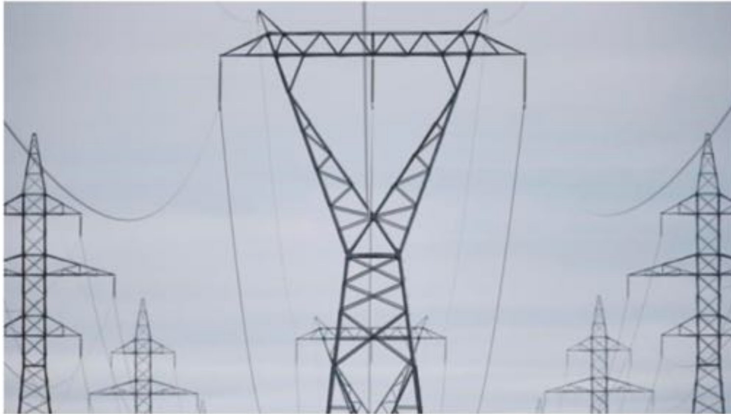
Manitoba Hydro power lines are photographed just outside Winnipeg, Monday, May 1, 2018. THE CANADIAN PRESS/John Woods
