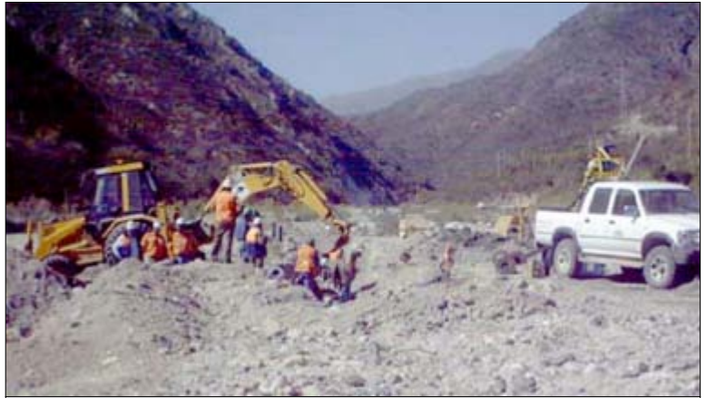
Crews clean up spill from Bajo La Alumbra mine slurry pipeline into the Villa Vil River in Argentina.
